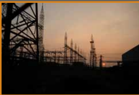
MAIN RECEIVING SUB STATION
